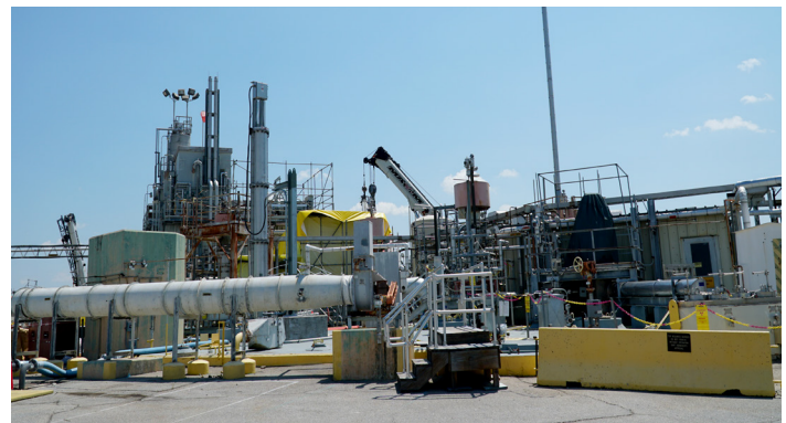
Crews with Savannah River Remediation recently completed modifications to convert Tank 42 into the third blend tank for Salt Waste Processing Facility feed. Pictured is the site of Tank 42.
