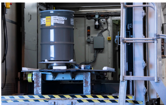
A transuranic waste drum ready for characterization in the RTR unit.
