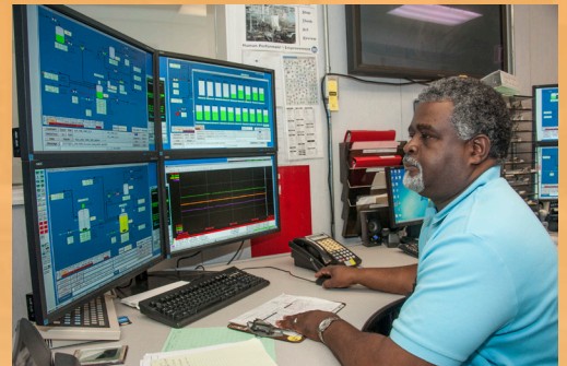
H Canyon operators check readings on the wall panel control system in the H Canyon Control Room (left); An operator works at the Distributed Control System, which controls many of the canyon processes (right).
